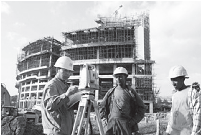
Picture 7: Chinese and Ethiopian workers were building the new African Union Headquarters in Addis Ababa, Ethiopia in November 2010. China picked up the US $200 million cost and the Ethiopia's tallest building was completed in 2011.
